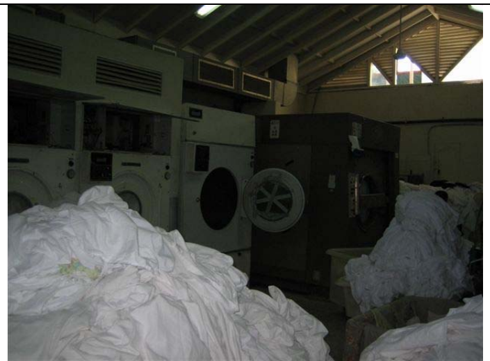
Picture 5.4 Beaches Negril Laundry - Dryers
