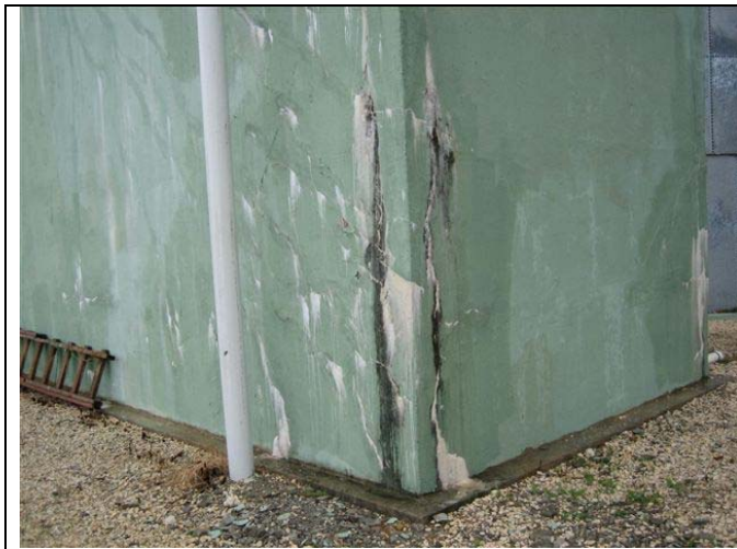
Picture 5.12 Sandals Whitehouse – Sewer Tank Failure
