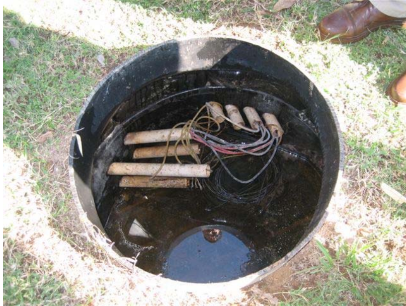
Picture 5.18 Sandals Whitehouse – electrical Manhole with Water
