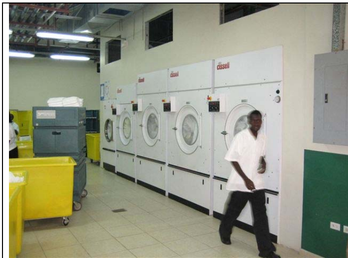
Picture 5.3 Sandals Whitehouse Laundry – Dryers
