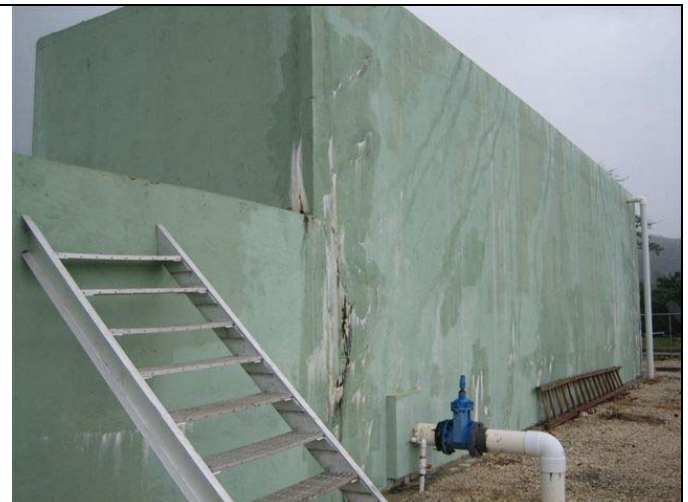
Picture 5.13 Sandals Whitehouse – Sewer Tank Failure 2
