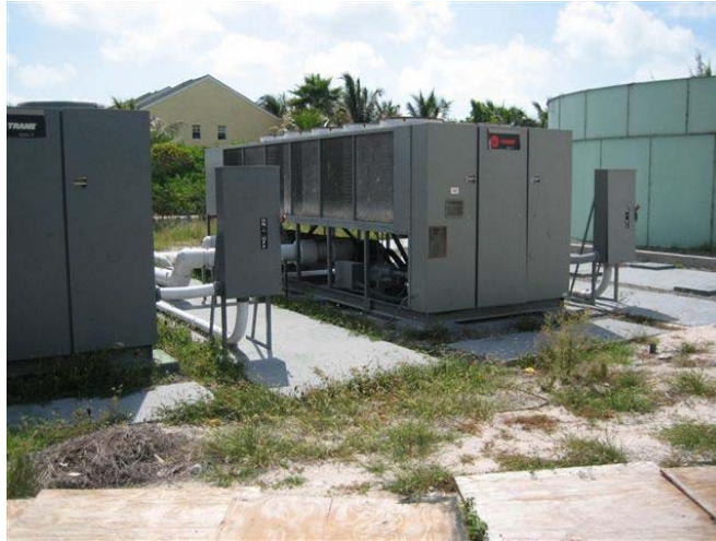
Picture 5.11 Beaches Turks & Caicos – A/C Chiller
