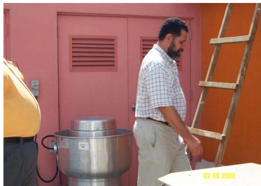
Picture 5.6 Sandals Whitehouse – Exhaust & Fresh Air Intake
