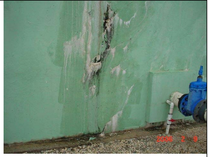
Picture 5.15 Sandals Whitehouse – Sewer Tank Failure 4
