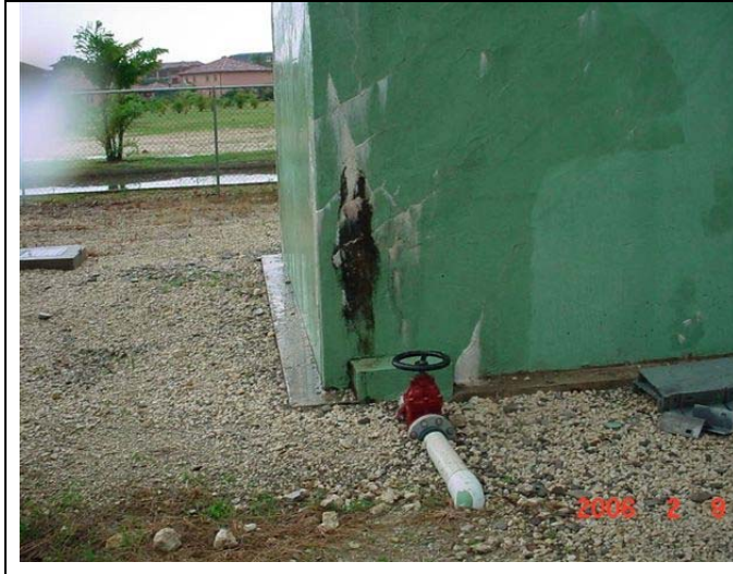
Picture 5.14 Sandals Whitehouse – Sewer Tank Failure 3
