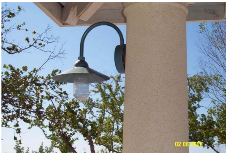
Picture 5.17 Sandals Whitehouse – Light Fixture Base not sitting properly on Column
