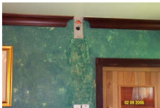
Picture 5.7 Sandals Whitehouse – Damp area on Wall from Air Conditioning
