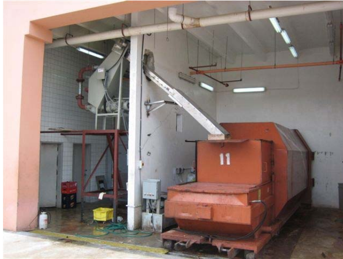
Picture 5.5 Sandals Whitehouse – Somat Garbage Disposal System
