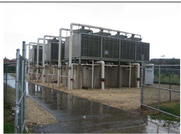
Picture 5.9 Sandals Whitehouse – Air Condition Chiller
